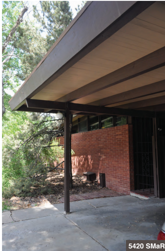
This brick masonry wall extends beyond the house to shelter a patio behind.
