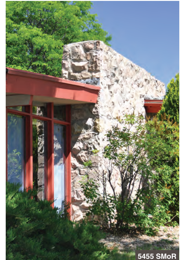
Here, the relationship between the secondary chimney volume and the roof and wall planes of the house are visible.
