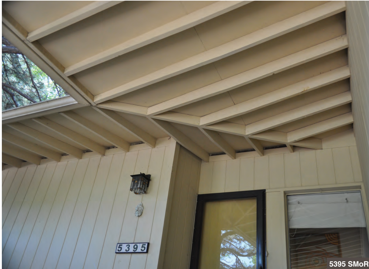
The roof planes of these two primary volumes join to shelter the primary entrance of the house. The exposed rafters form this decorative detail above the front door.
