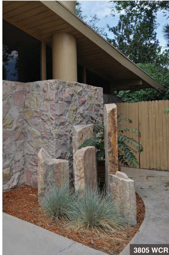
The rhyolite masonry of this chimney stops short of the roof line. A round concrete flue rises above it, in front of an inset window composition and behind the roof fascia.
