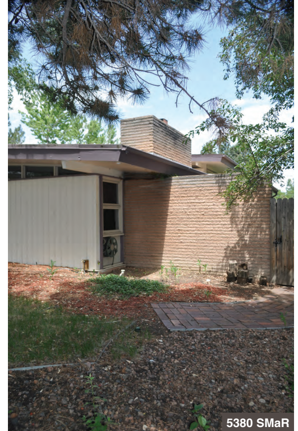
This roof plane projects beyond the side of the house, wrapping around the chimney and resting atop an extended masonry wall.
