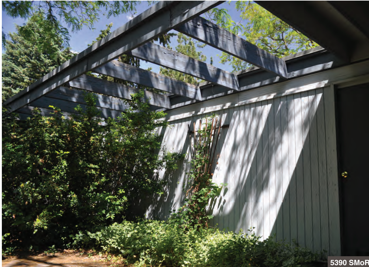
Open roof planes also appear. This arbor is designed as an extension of the garage roof. It serves as a sunscreen for the patio below.
