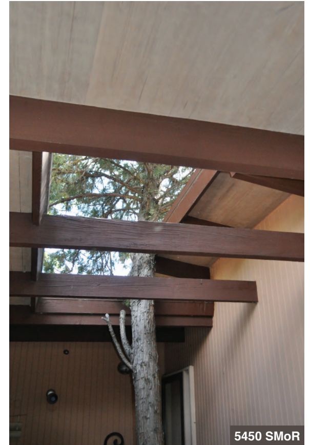
Where additional natural light is desired, like this deeply recessed entrance courtyard, the roof deck is removed. A pine has been trained through the opening.
