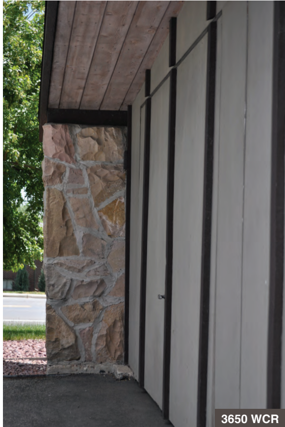
The wall and roof plane project the same distance beyond the face of the house, creating more privacy and shelter.
