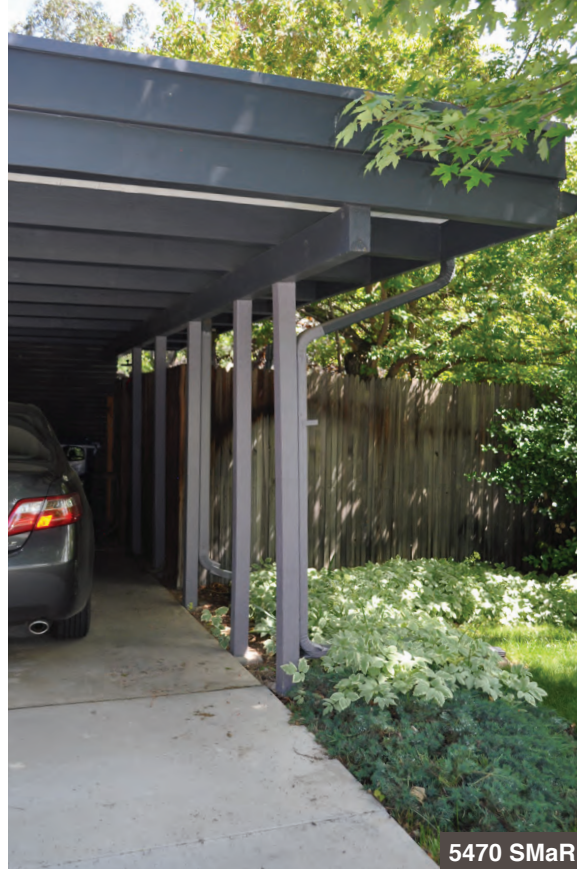
On this carport, the roof plane projects over an open wall plane formed by a series of wood columns.
