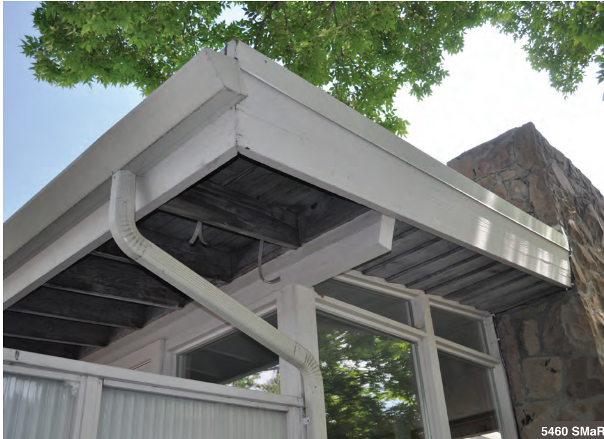
Rafters running parallel to the fascia, at right, are concealed above a lapboard soffit. At left, like the beams, they're exposed.
