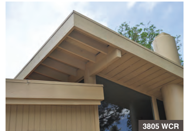
A similar detail appears above. The rafters are exposed at left and concealed at right, where the round concrete flue of the chimney penetrates the roofline.
