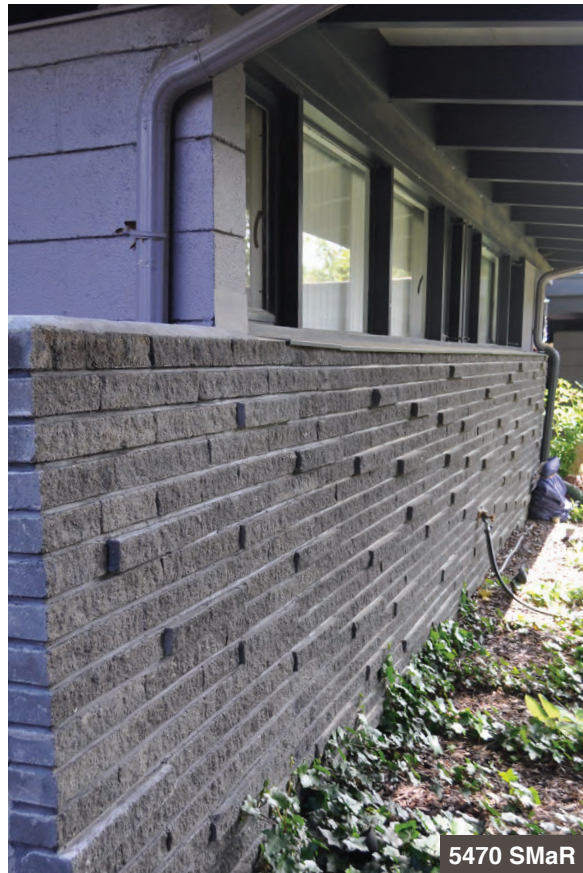
Front and side wall planes often project beyond adjacent walls into the landscape.
