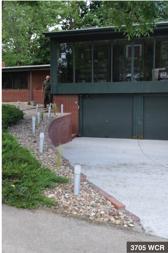
This curvilinear retaining wall follows the driveway as it drops to a garage located below street grade.
